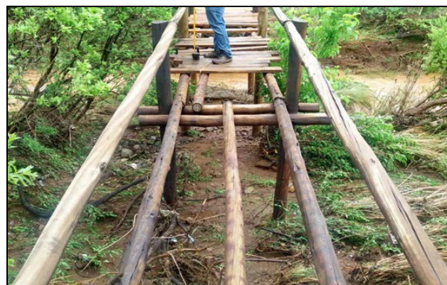
The bridge seen from the eastern bank of the Moreletaspruit, without its walking surface, during the repair process.
