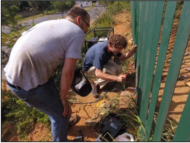
Thomas Schmidt (left) and Ralph Enslin (right), welding a slat back into place in the FGNR's palisade fence along January Masilela Ave.
